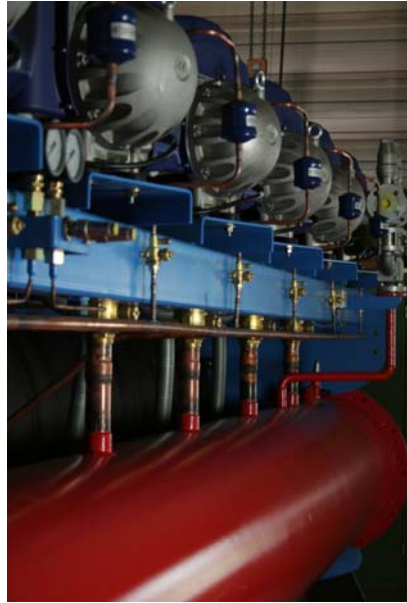
Axima 1800kW Watercooled Chiller
